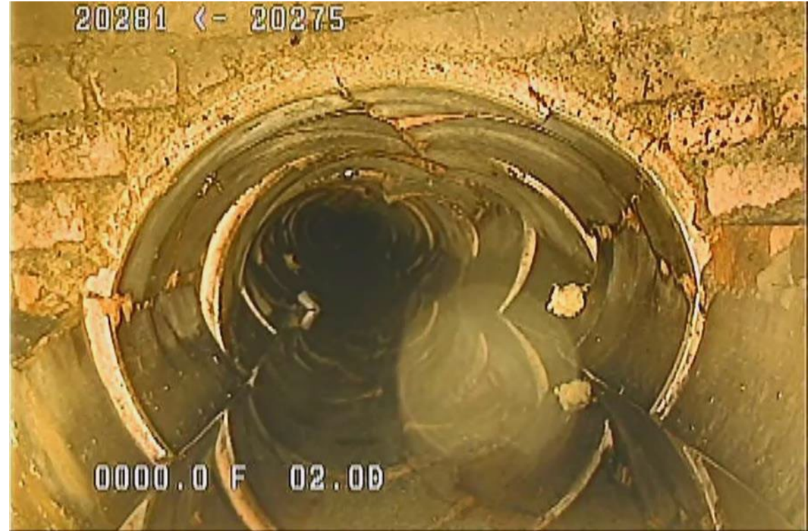
Deformed Pipe on Pierce St.
