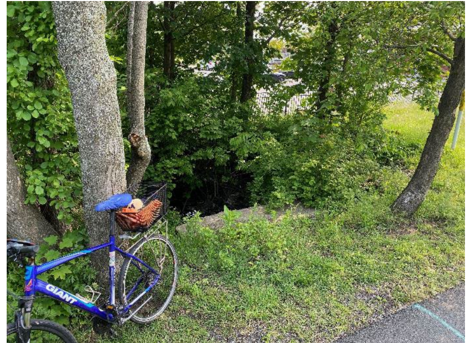
Overgrown Culvert along Bike Path Near CVS
