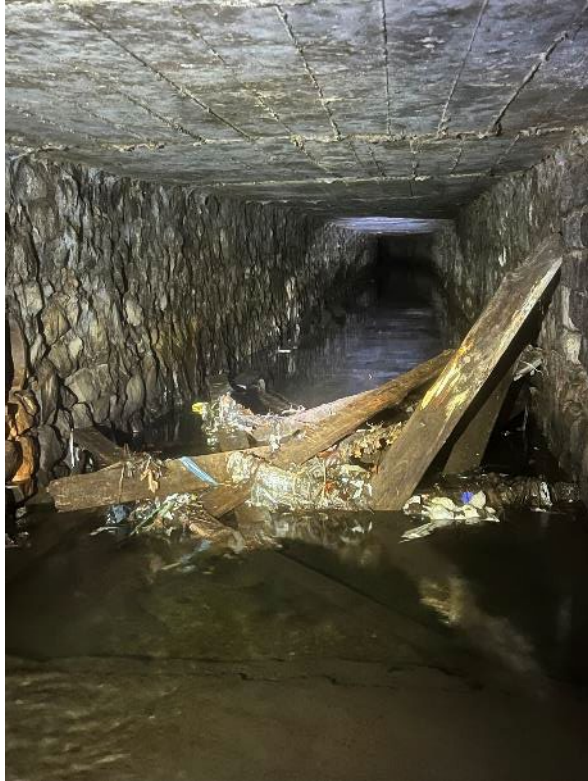
Pile of Debris in Edgeworth Brook Culvert near Russell St.
